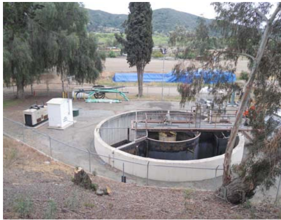
Existing "B Plant" Lift Station
