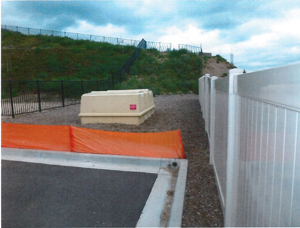
Pressure Reducing Station at Olive Hill Estates
