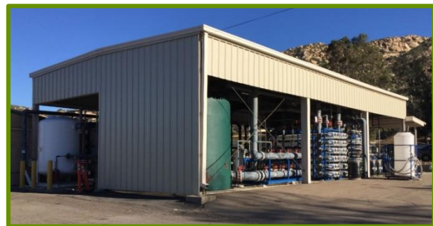
Completed reverse osmosis system upgrade for RMWD
