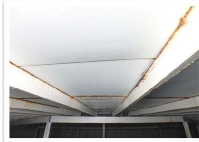
Roof Interior (rust) - from 2025 USG Inspection Report
