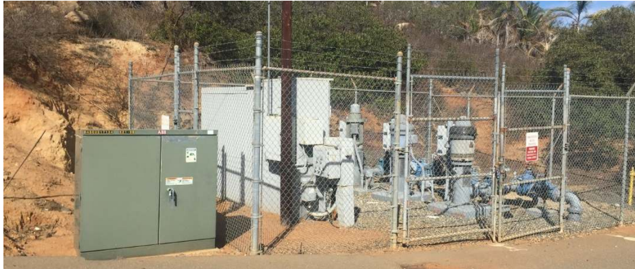
Pump Station U1
