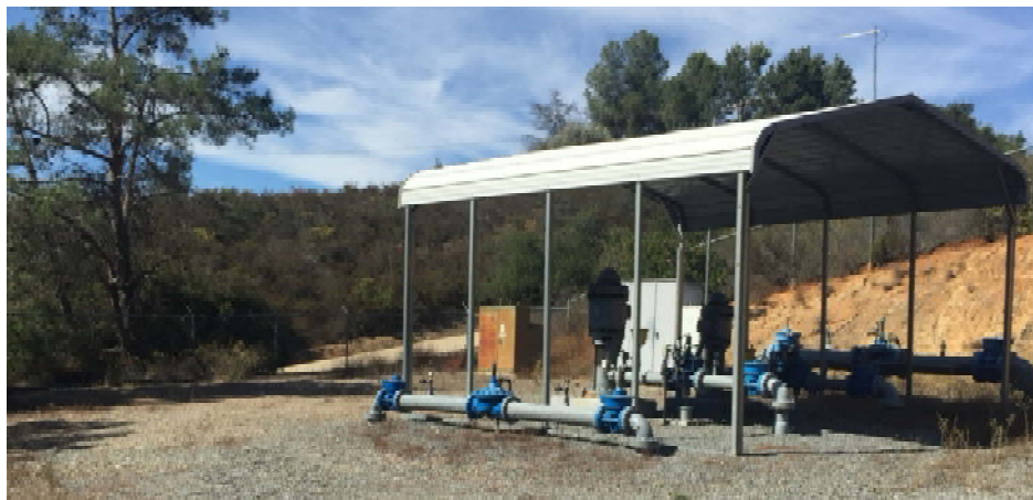
Pump Station McGee
