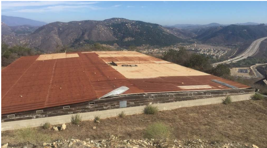
Sumac Hill Reservoir
