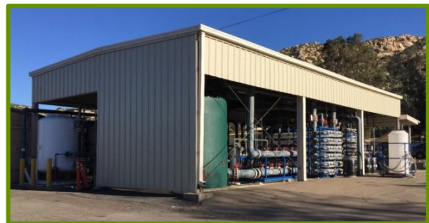
Completed reverse osmosis system upgrade for RMWD
